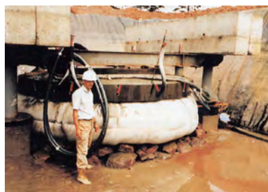
Test Rig Showing a Filled Unit
