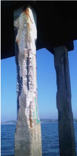
Fig. 8 - Damaged R.C. Pile, Hunterston
